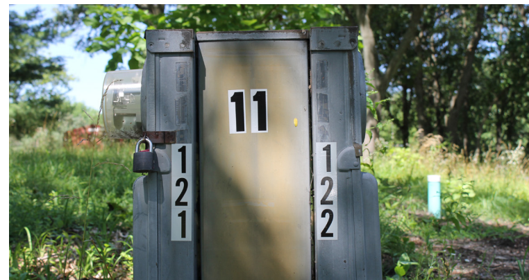
Here is the pedestal with the refreshed numbers and the Section identified in the middle. The section numbers are 3-inch vinyl reflective and the lot numbers are 2-inch vinyl reflective. These were purchased at Woody's True Value Hardware Store.
