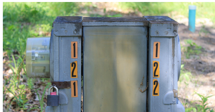
Original Section Numbers Located on Electric Pedestals
