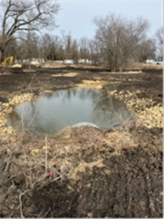
Figure 1 shows finished stream restoration section below culvert under Woodhaven Drive East looking at the area between sections 8 & 9. This created pool will act to slow water down thus reducing its erosive force.
