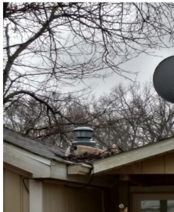
Figure 4 Can you see the goose nesting on top of this roof? This shows how difficult it is to locate nests out on property.
